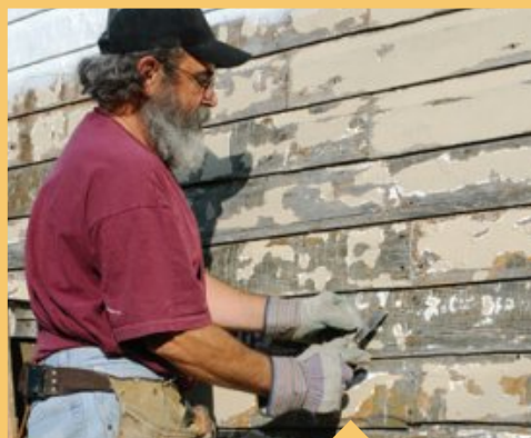
⊘ Unsafe home repair
